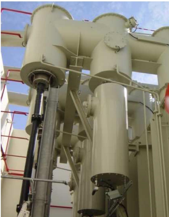
Fig. 11. GIS surge arresters to protect gas insulated switchgear
