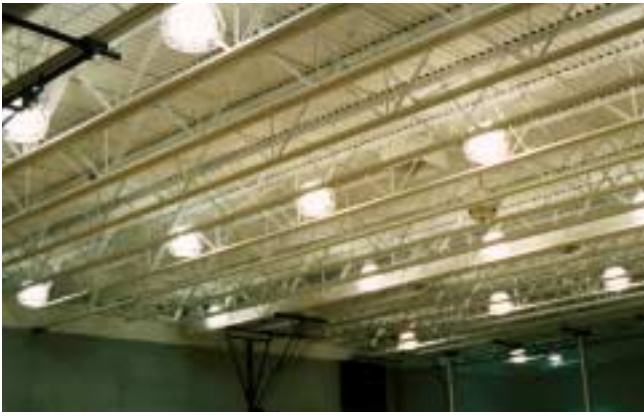
Figure 13-28 Unprotected open web steel joists present a large surface area to absorb the heat of a fire, expand, and collapse. Structural steel will lose 50 percent of its strength at temperatures of 1,000°F.
