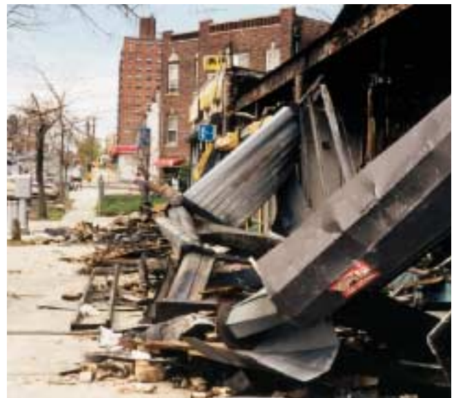
Figure 13-33 This is the scene of a typical “parapet” wall failure common in Type III ordinary construction.
