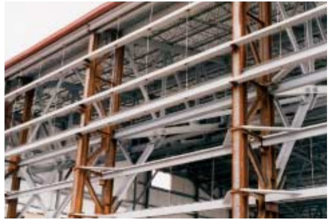
Figure 13-16 Buildings of Type II construction will have structural elements with little or no protection from the effects of fire. Remember, in the event of a fire, these unprotected steel structural members may fail and collapse with little warning.
