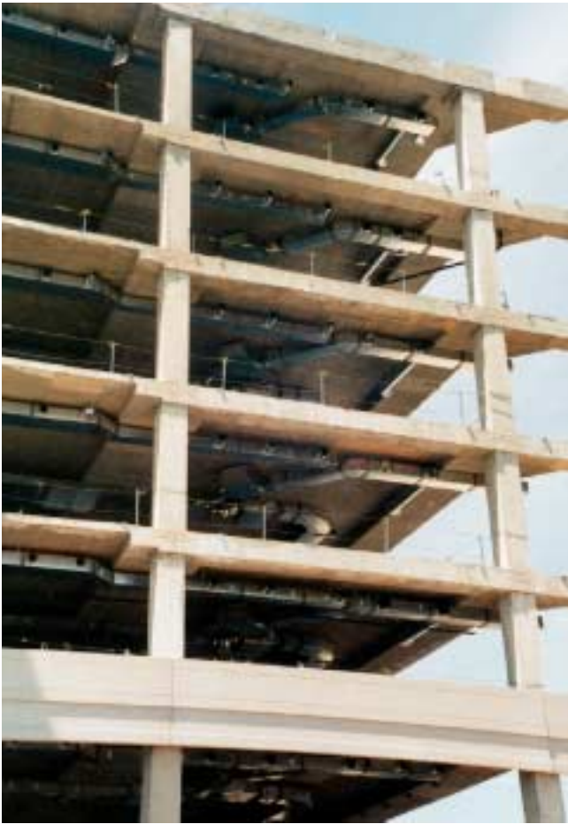
Figure 13-15 A typical Type I building, with structural members designed to resist the effects of fire for three to four hours. This building is of reinforced concrete construction.
