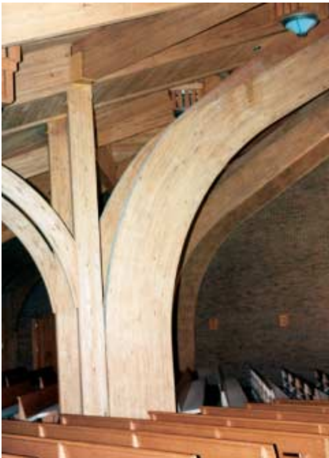
Figure 13-19 Type IV buildings, heavy timber construction, have large wood structural elements with great mass. The mass of these structural members requires a long burn time for failure. The connections, usually steel, are the weak points in this type of construction.
