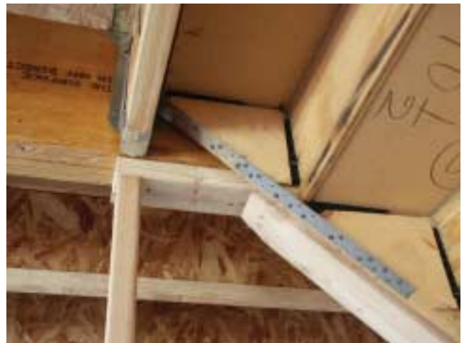
Figure 13-32 This prefab stair assembly is hung in place by thin metal strapping. Note the staples and plastic shims that can quickly fail under fire conditions.
