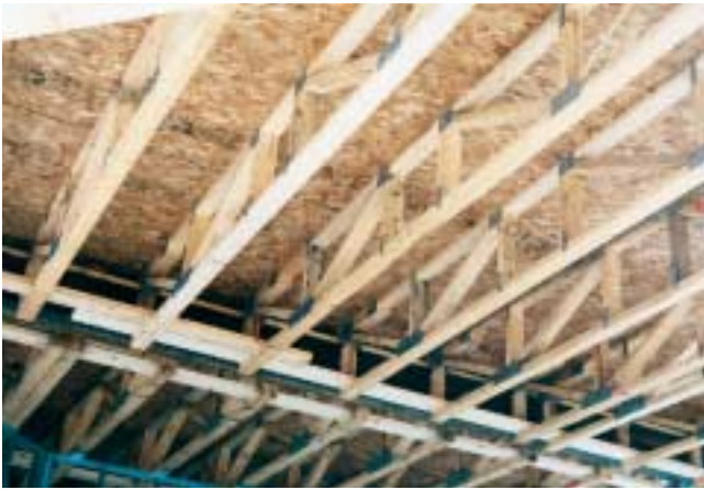
Figure 13-26 Wood trusses provide a large surface-to-mass ratio, fuel load, and void spaces—three of the worst conditions a firefighter will encounter during structural firefighting operations.
