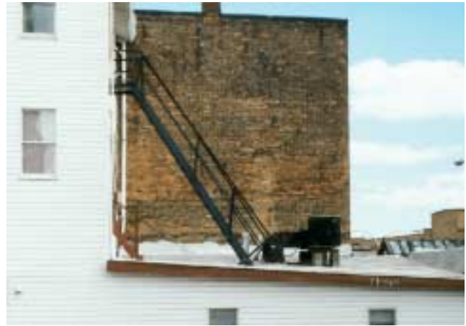
Figure 13-2 The steel stairs and air-conditioning unit apply a concentrated load on this roof structure. Also note the potential instability of the air-conditioning unit placed on cement blocks.
