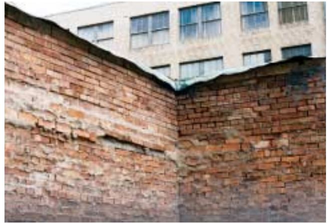
Figure 13-9 Prior to a fire, the effects of age will take their toll on masonry walls. How stable is this wall with joint deterioration and lack of full mortar bond?
