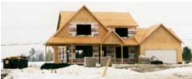
Figure 13-21 The wood frame structure, Type V construction, is the most common type of construction in North America.
