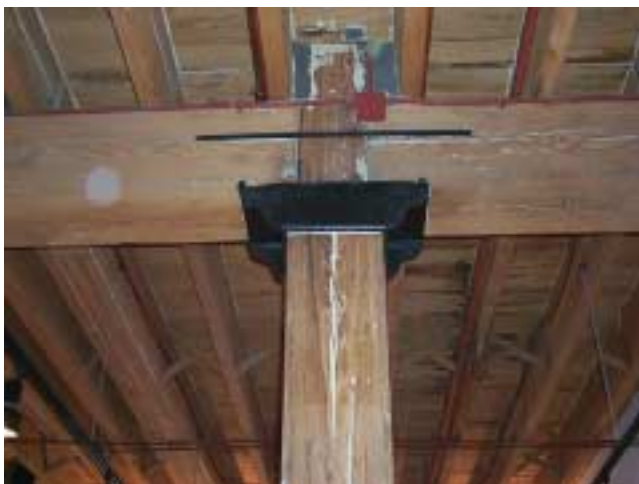
Figure 13-8 This column is supporting a beam, flooring, and another column. Columns are subjected to compressive forces.
