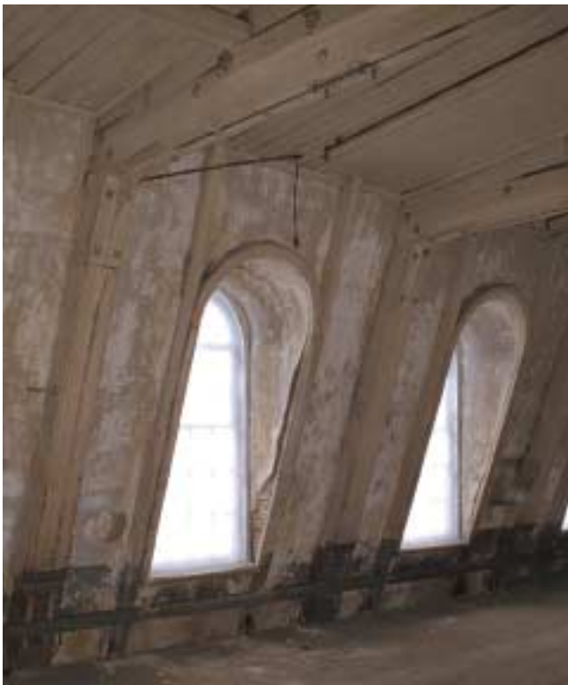
Figure 13-31 An internal view of dormers in a mansard roof. Fire can run through the many voids between the exterior and the roof.
