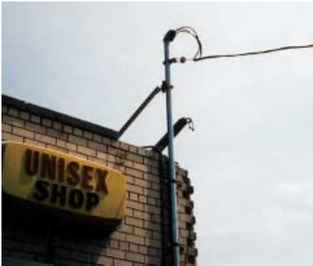
Figure 13-34 This electrical service entrance and weather head may be the eccentric load causing an early failure of this parapet wall.
