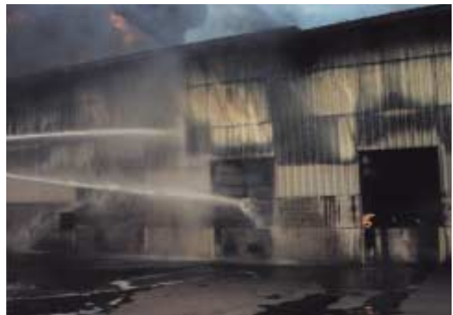
Figure 13-4 This ladder pipe operation is applying an impact load to the wall of this structure. As the wall weakens, it will eventually collapse. (Photo courtesy of William H. Schmitt, Jr.)
